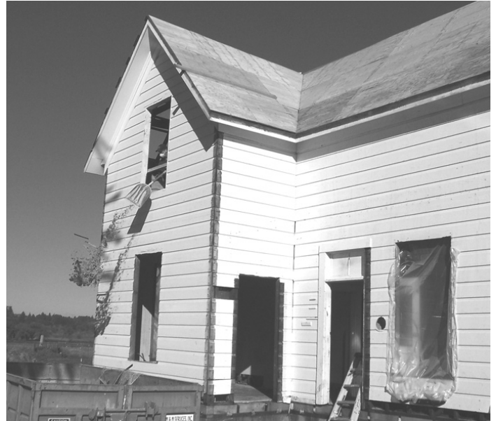
A volunteer workday for interior demolition of the second floor. Photo: Wayne Mitchell
